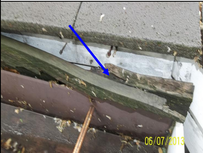
Photo 2 – Fascia board that has rotted and no longer can support the gutter. The gutter is severely dislodged from fascia board.
