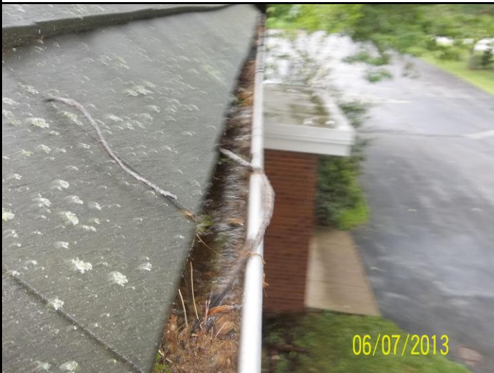
Photo 3 – Gutters are filled with debris and not draining properly.
