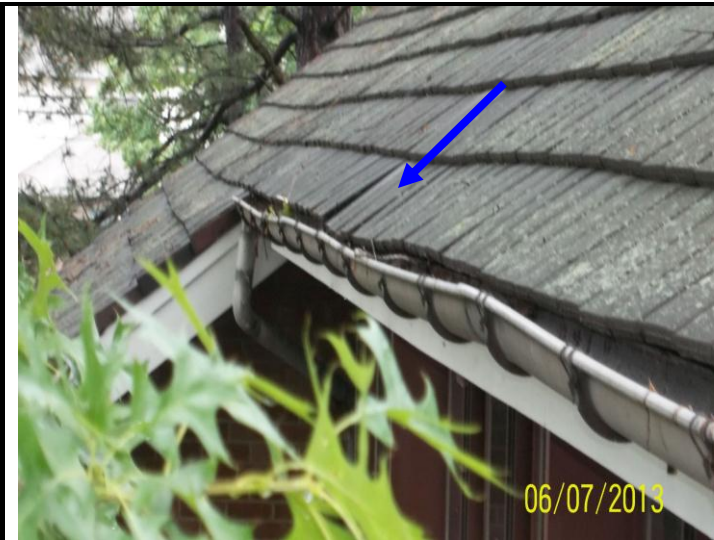
Photo 1 – Area of rotted wood deck on Sanctuary roof.
