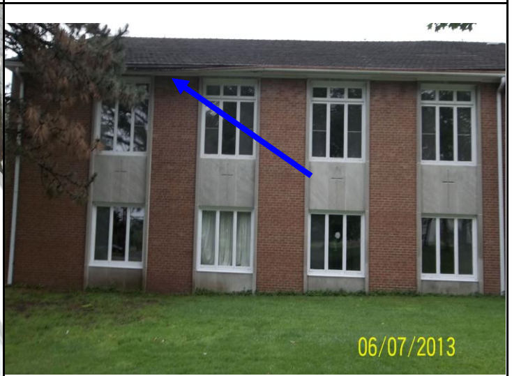
Photo 4- Fascia board has rotted and can no longer support the gutter.
