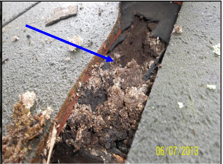
Photo 1 – Rotted wood deck. Cement tile has split with lack of deck support.
